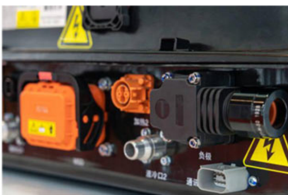
BATTERY PACKS BMS
